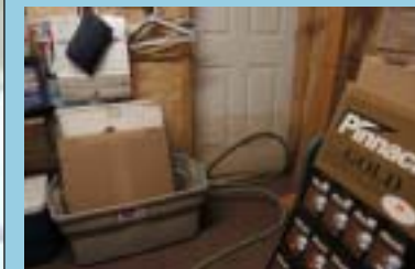
Decatur County, TN, May 20, 2003 -- A waterline caused by the flooding of the Tennessee River is clearly visible in the pro shop of a local golf course. Photo by Mark Wolfe/FEMA News Photo
